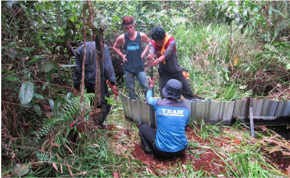
Figure 4. The project team piloting a dam design on a small former 'logging' canal.
